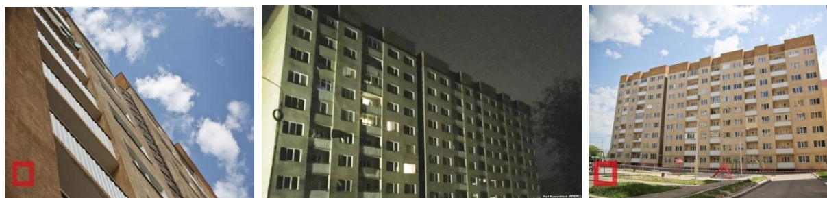
Figure 1. Tilting high-rise buildings of the Zerdeli microdistrict in the Algasbas district of Almaty city
