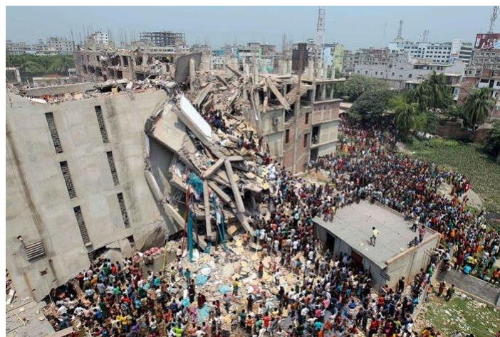
Figure 4. The process of collapse failure of the 8-storey building of the commercial and industrial center Rana Plaza in 2013
