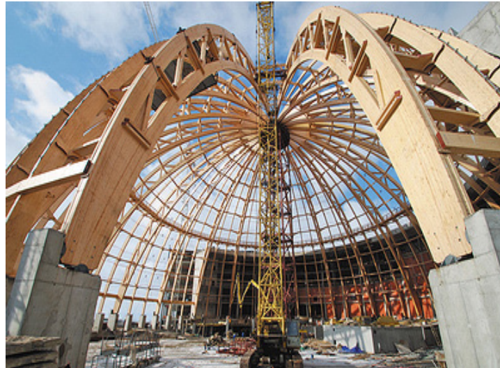
Figure 1. The ribbed dome of the water park with a diameter of 90 m
