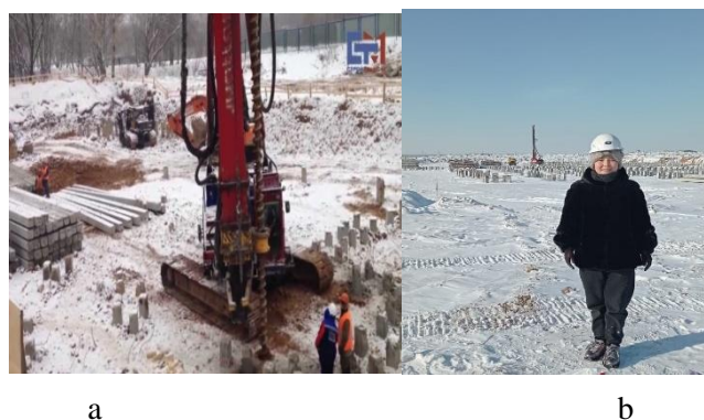
Figure 1. Fragments of the device of pile foundations in seasonally frozen soils: a – work on preliminary drilling of seasonally frozen soils in the places of pile driving; b – driving of a reinforced concrete pile into seasonally frozen soil in Nur-Sultan
