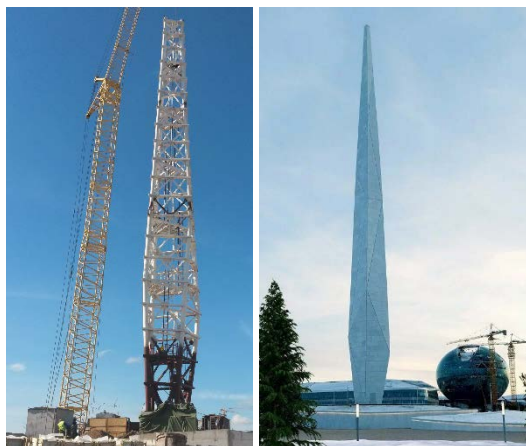
Fig. 1 70 m high monument in Nur-Sultan, Kazakhstan. a) Structural backbone, b) Finished structure with cladding
